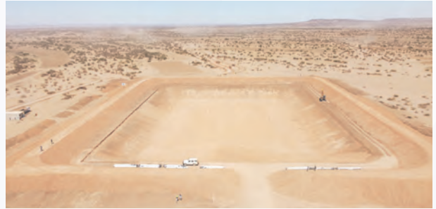
Aerial footage of the construction of Ijaara Hafir Dam (132mX92mX6m) with storage capacity 57,863.00 cubic meters. This dam is located in the South East region of Gabiley, Somaliland.
